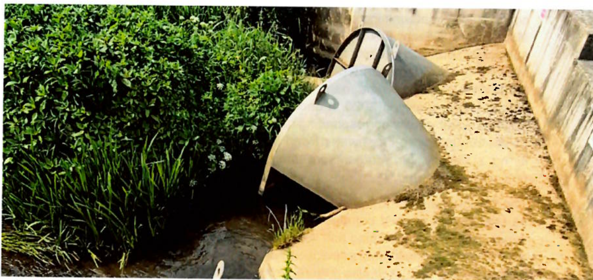
Figure 2-1. Inlet conditions on Vortex Flow Control Structure on a UK EA flood scheme (typical low flow conditions).
