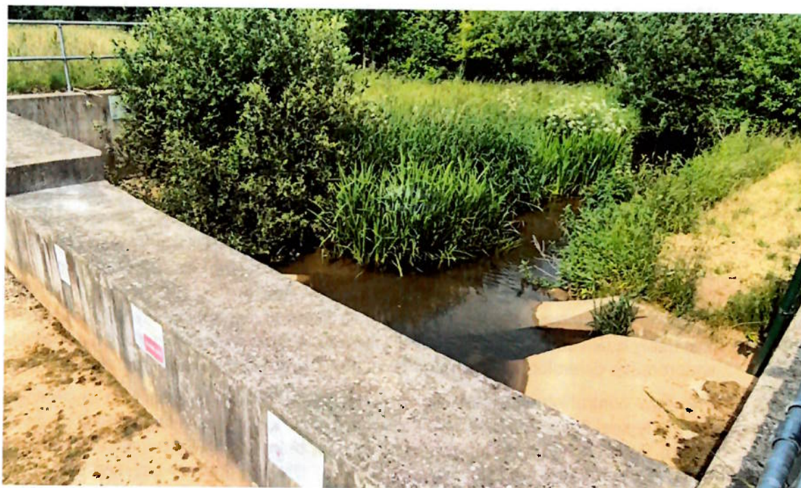
Figure 2-2. Outlet conditions on Vortex Flow Control Structure on a UK EA flood scheme (typical low flow conditions).
